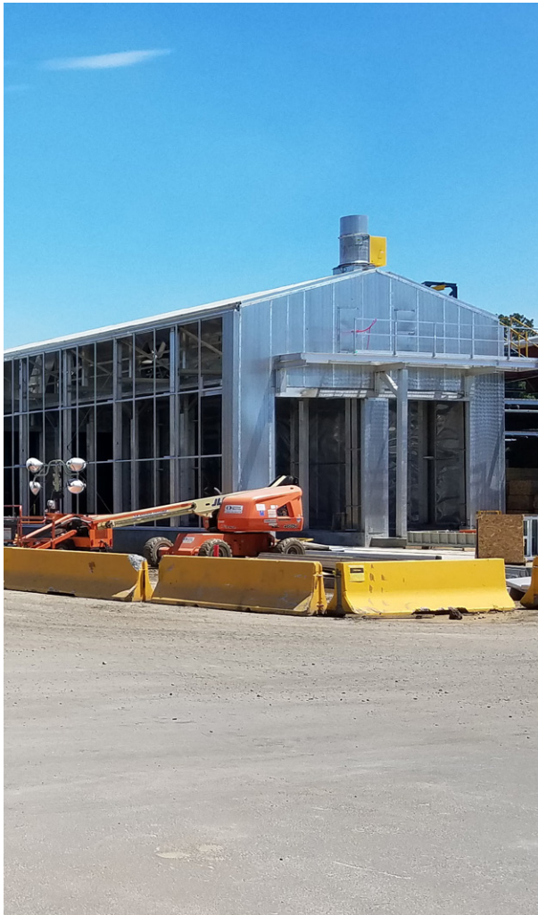
The new continuous kiln at Meldrim has a drying capacity of 107 million board feet a year. Improved drying quality will also lead to better grade outturns.
